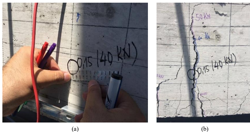
Figure 13. Measurement of crack width: (a) In-situ crack gauge measurement at 40 kN; (b) Detail view of vertical flexural cracks in the tension zone
