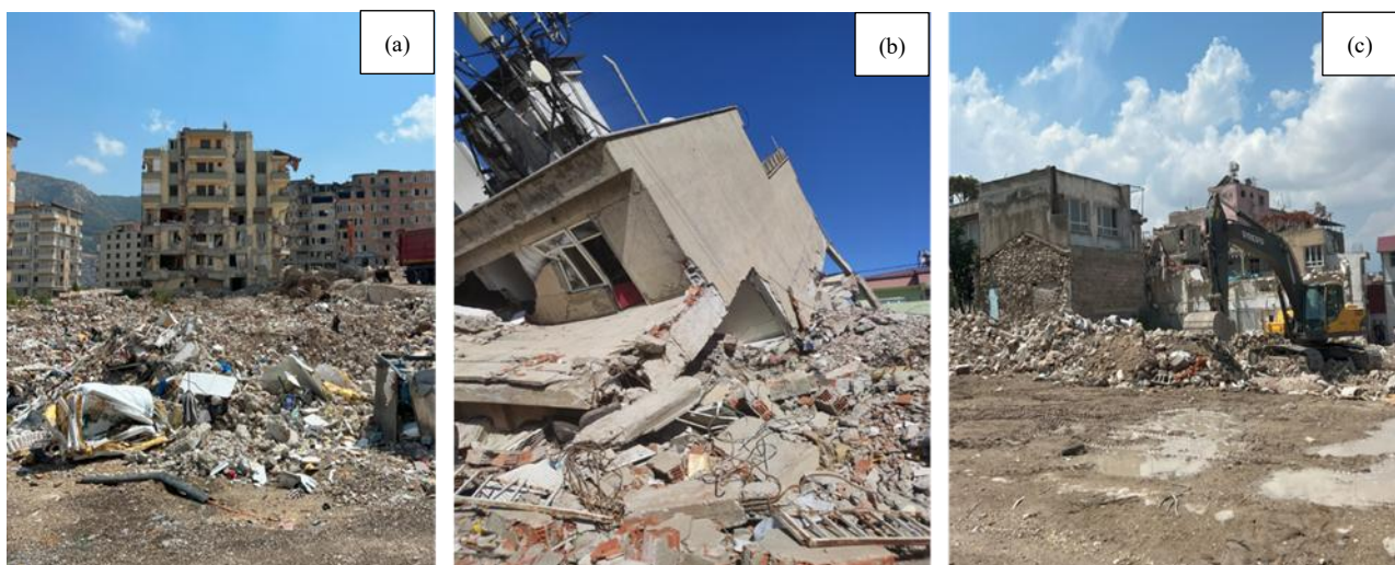
Figure 14. Debris clearance and selective demolition in dense urban fabric: (a) mixed debris fields adjacent to occupied blocks; (b) partially overturned reinforced-concrete frame with rooftop equipment; (c) mechanical demolition and haul-off along a constrained street.
