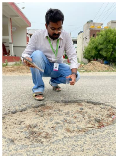
Figure 13. Field measurement of pothole’s depth
