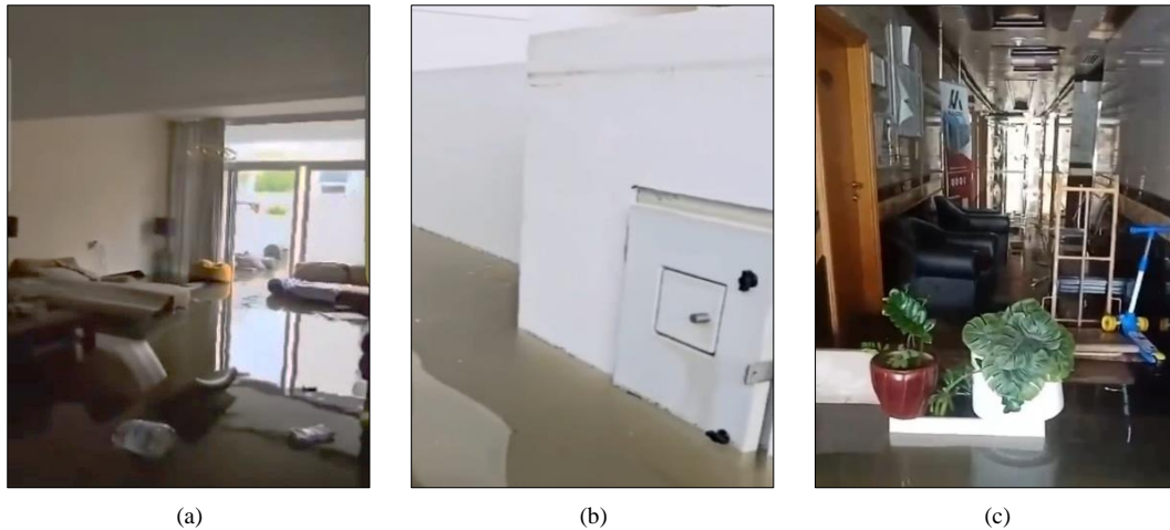
Figure 9. (a) Water ponding inside house, (b) Water ponding inside house boundary, (c) Water ponding at lobby
