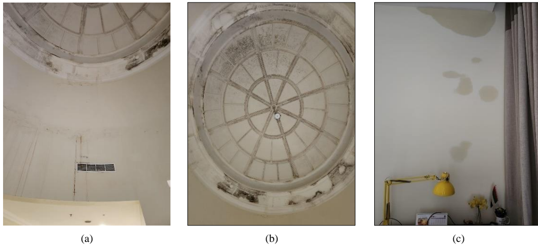
Figure 7. (a) Water leaks at ring beam, (b) Dampness and Fungus, (c) Dampness in wall
