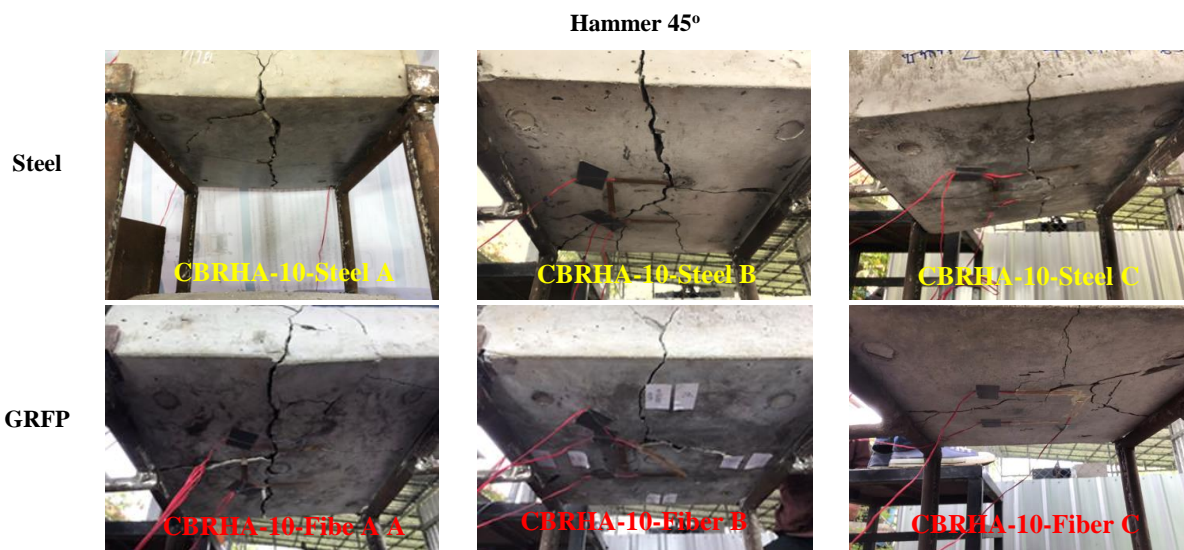
Figure 11. depicts the damage patterns from impact on steel-reinforced and fiber-reinforced concrete using a - 45 degree angled hammer head
