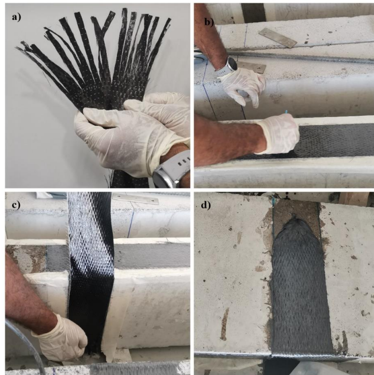
Figure 6. Steps of Alternative U-wrap Installation a) CFRP fabric cut at ends b) Installation of CFRP soffit laminate c) Installation of end anchors d) The flared ends of the anchor inserted to the precut holes at beam sides
