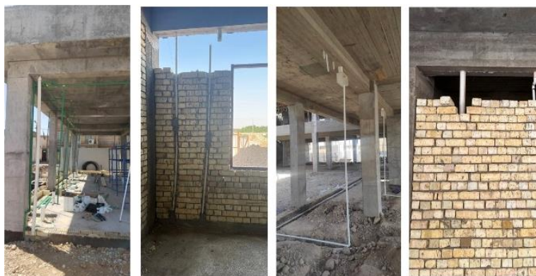
Figure 1. Vertical services pipes (school building/Iraq)
