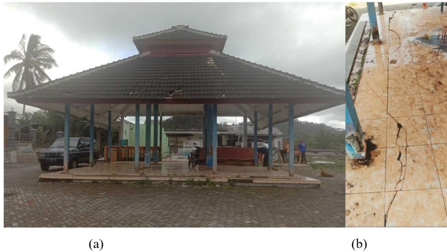
Figure 5. (a) Demolished homes surround the state of hamlet hall. The structure that collapsed due to the earthquake on April 10, 2021, has not yet been reconstructed (June 2022). (b) Cracks occurred on the hamlet hall floor due to the April 10, 2021 earthquake.
