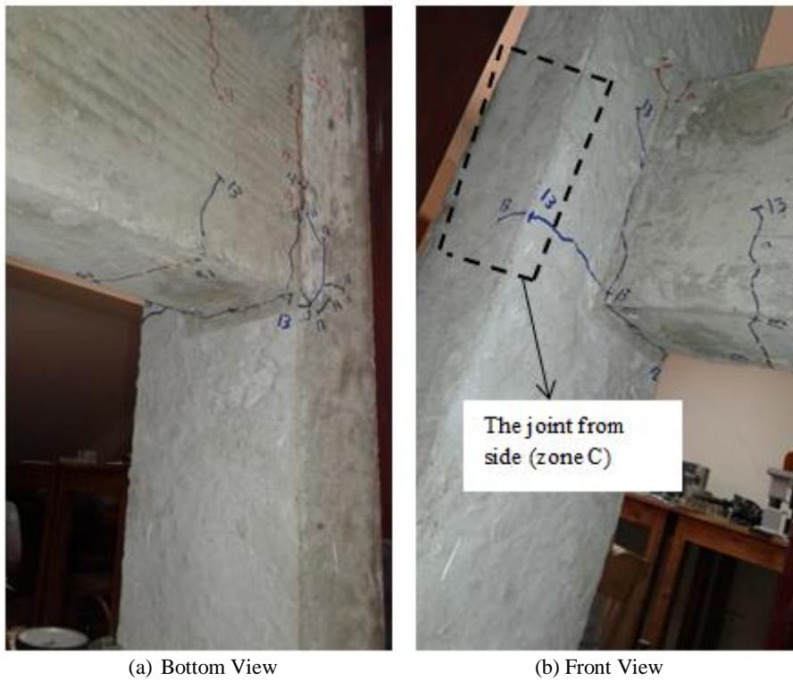
Figure 10. Crack pattern of specimen after the 2 nd cycle ending when the load toward upward
