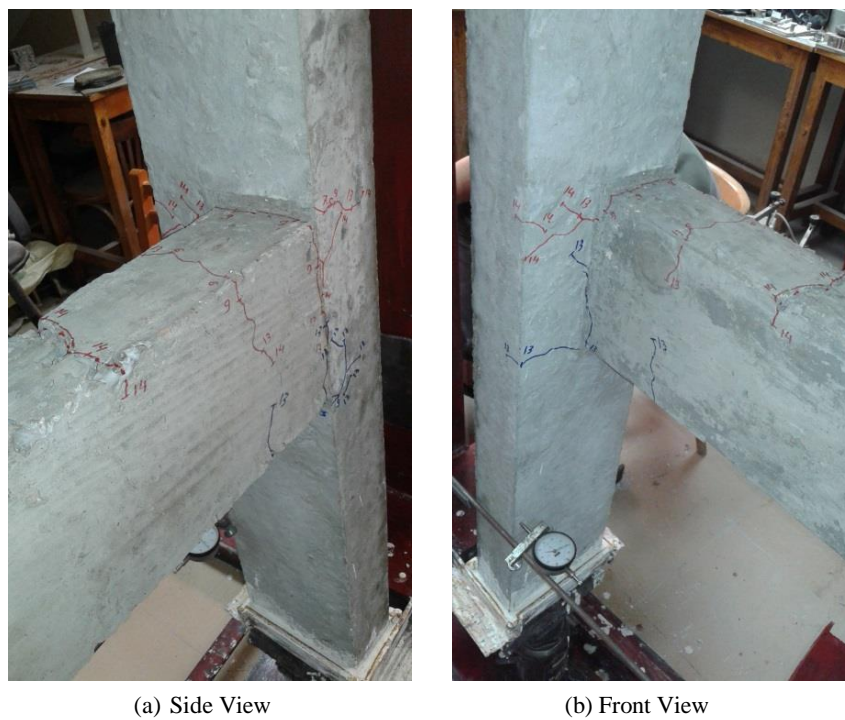
Figure 11. Crack pattern of specimen after the 3 rd cycle ending when the load toward down ward
