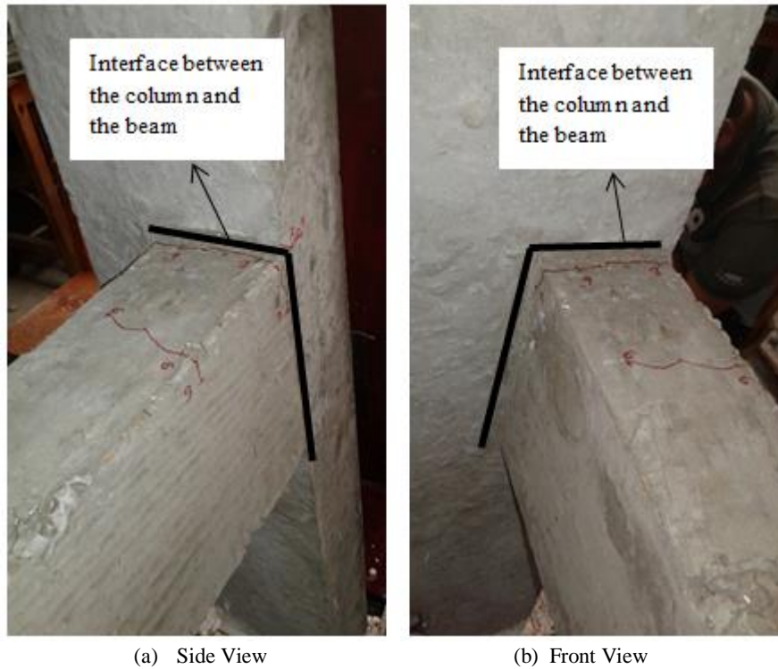
Figure 8. Crack pattern of specimen after the 1 st cycle ending when the load toward down ward
