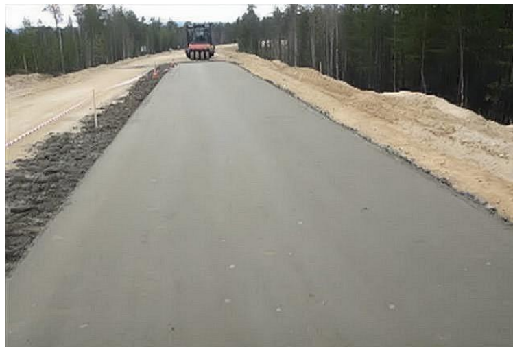
Figure 7. Construction of a pavement of reinforced soil on an oilfield road in the Murmansk region K-V-PP "Lotta"
