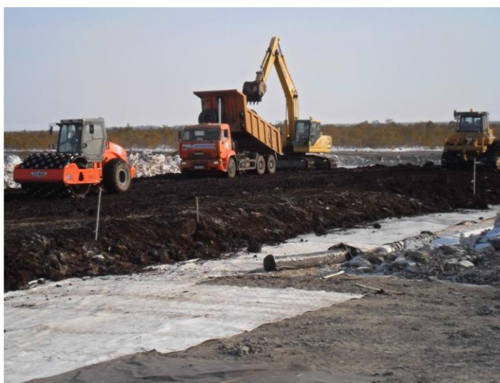
Figure 6. The construction of the lower part of the embankment from frozen ground in a holder made of geosynthetics with a heat insulator (N-Urengoy, Pestsovoe deposit)
