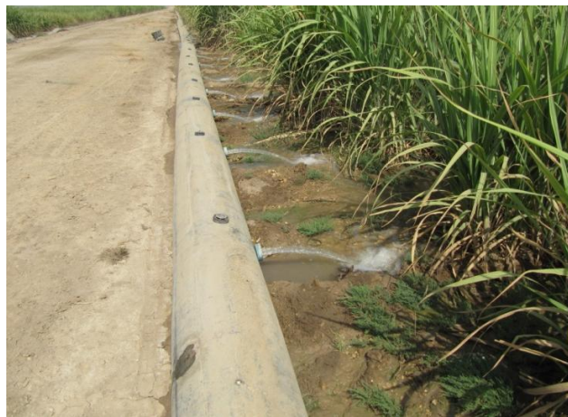
Figure 2. Hydro-flume with Adjustable out-let valves
